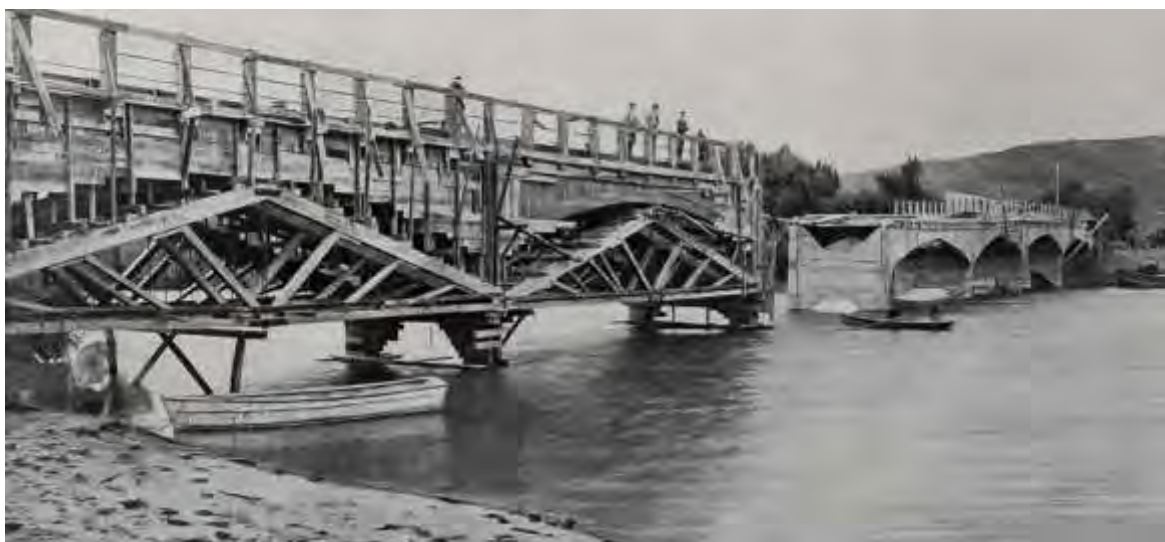
On the Great East Coast Railway Route: The new ferro-concrete bridge now under construction over the Whakatāne River, Bay of Plenty, 1909. Source: Sir George Grey Special Collections, Auckland Libraries, AWNS-19091021-4-4
