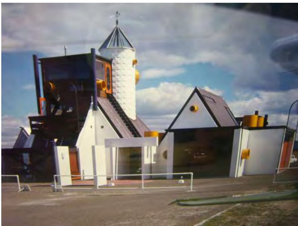
Photograph of terminal under construction Source Archives NZ Reference No. AEPK W2774 20231 Box7
