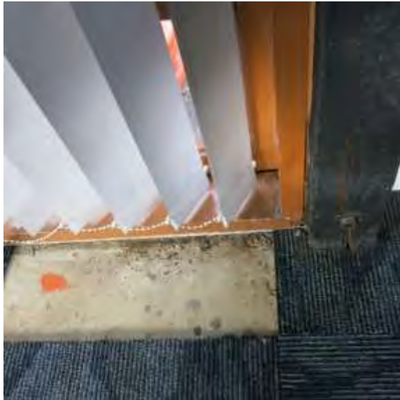
Showing water damage in main lounge (left) joinery detail
